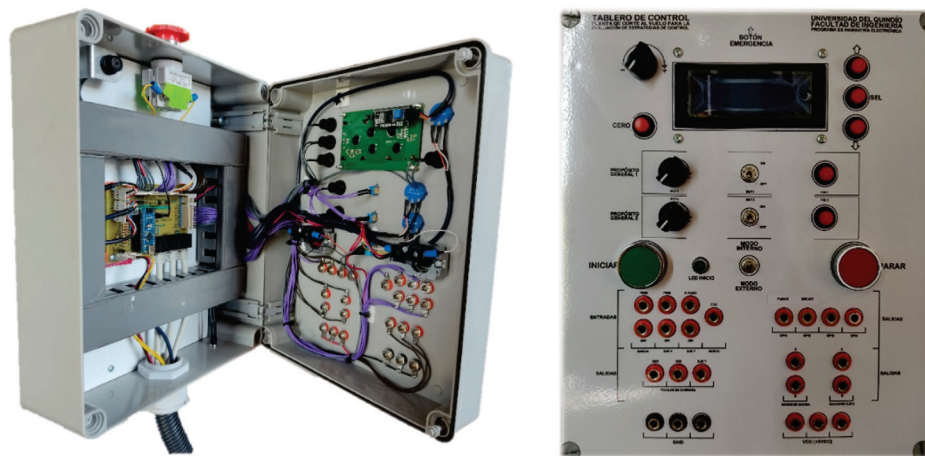
Figure 21. Control panel for the flying-cutting plant. Electrical circuits - left, graphical user interface - right
