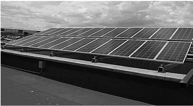
Figure 4. Installed solar panels Source: Taken from fieldwork.
