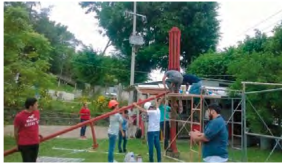
◀ Figures 53 to 63. Next, the cable poles are connected to the central members that articulate the movement of the transformable system; each connection is made in symmetry to compensate for the weight of the structure.
