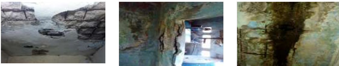
Fig. 2. Elements showing the corrosion of steel.
