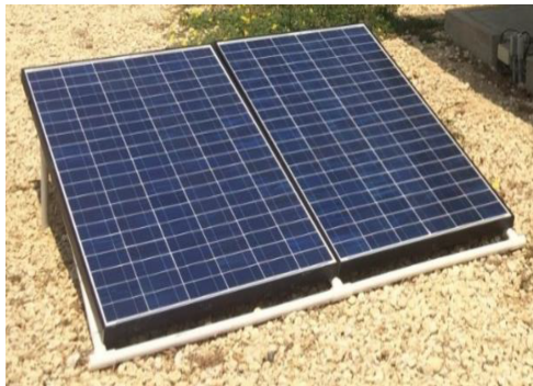
Figure 1 Installation setup for the PPs with 11^\circ tilting orientation south
